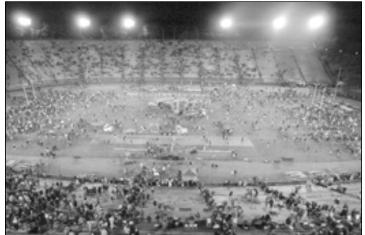
Fans joined excavators on the field following the Stanford-Notre Dame game for the beginning of the demolition of Stanford Stadium.
